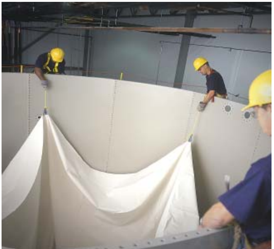
▼ After securing the base, the 600-lb-per-sq-in.-tensile-strength slick liner is pulled up and secured over the top prior to installing the silo cover. SHICK
